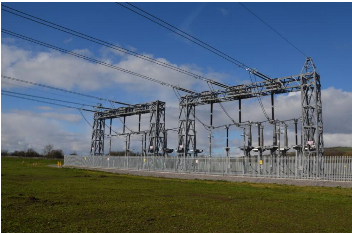
Image 4.12 Example CSE compound with gantry 20
